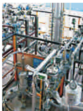
Safety and control valve rig to feed various incineration nozzles/lances
