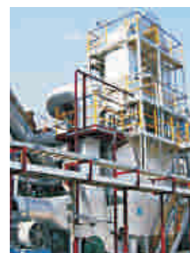
Flue gas treatment with DeNOx unit and economizer
