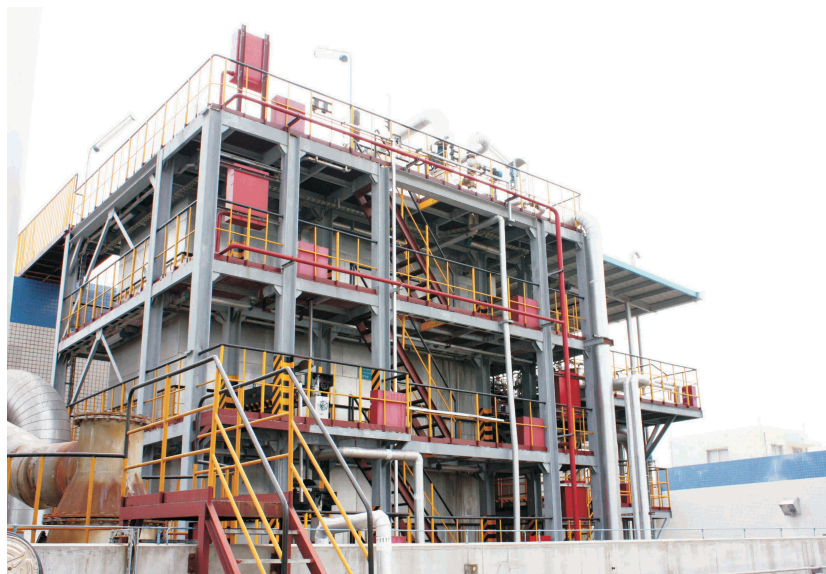
Steam boiler after waste incinerator
